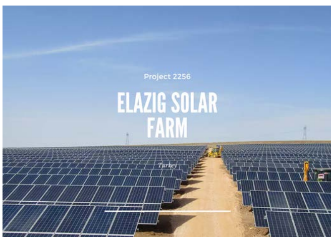
Project 2256: Elazig Solar Farm in Turkey
